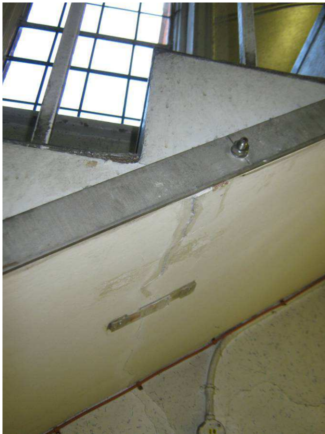
Photo 12. Cracking to soffit of staircase
